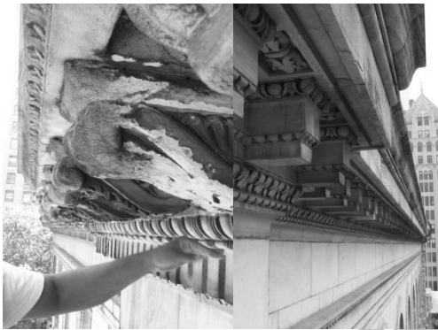
Figures 5a and 5b. Deteriorated modillions at main cornice without drip groove (left) and sound modillions at high cornice (right) with drip groove.
