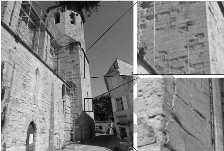
Figure 1. Spalling of dimensional stones on the southern façade of Saint Maurice Church (14 th century) buildup with Yellow and Grey Caromb stones in Caromb, Vaucluse, France.
