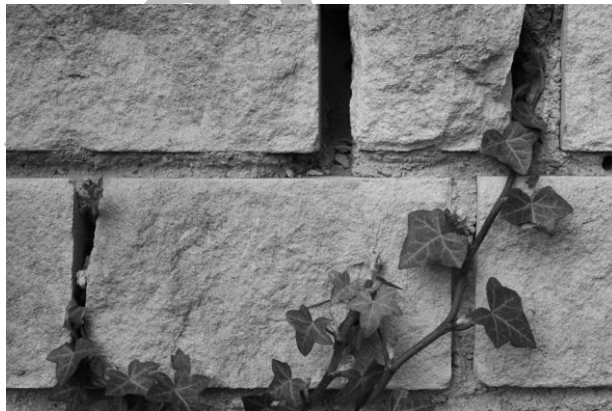
Figure 1. Ivy shoots exploiting defects in test wall, Wytham Woods, near Oxford, UK.
