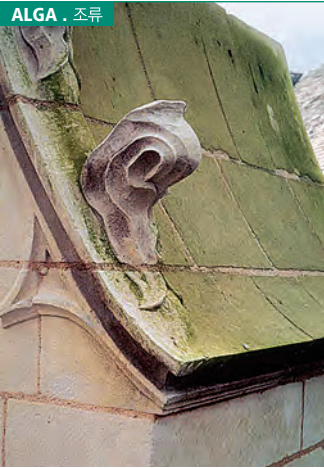
Green algae growing on a limestone buttress. 석회석 부벽의 녹조류
